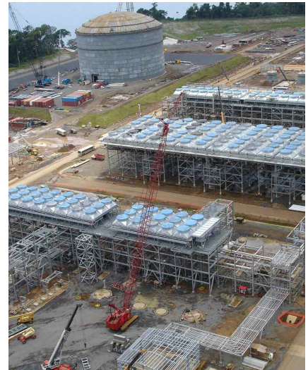
INTEGRATED APPROACH The recently completed Equatorial New Guinea LNG plant, shown here under construction in 2005, utilises a unified infrastructure to support telecommunications, business networking, control systems networking, access control and surveillance Stratos
